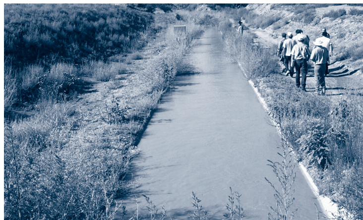
Parciantes of the Acequia de La Joya tour an acequia improvement project done in cooperation with the ISC Acequia Program and the U.S. Army Corps of Engineers.
