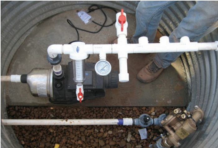
Figure 10-2. Sample inline pumphouse with spin filter manifold
